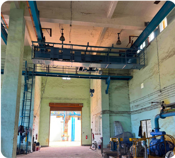
UNDERSLUNG EOT CRANE
